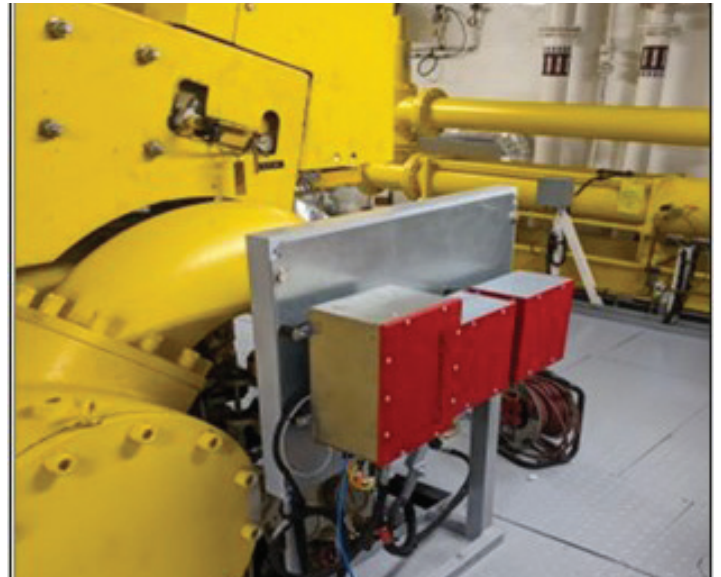
Figure 3: Installation on Marine Diesel Engine with chemical composition, Viscometer and Wear Sensors.
